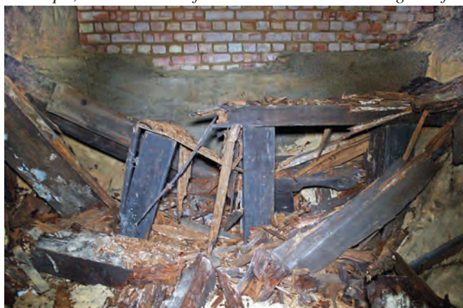
Decayed remains of the spectators' wooden seating
